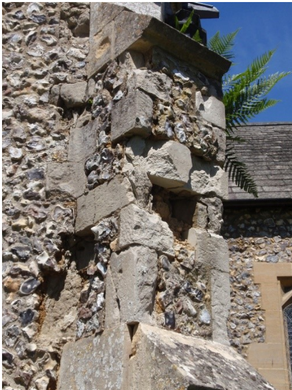
Repairs to the buttress on the SE corner and parts of the stonework on the roof
