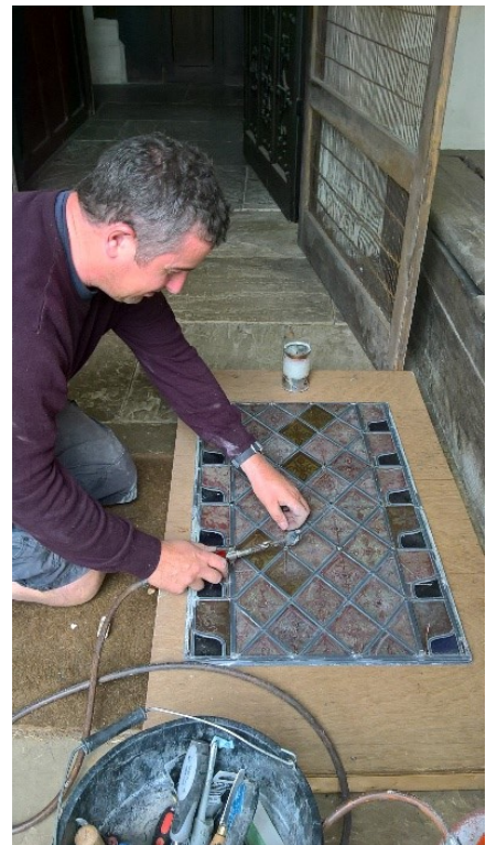
Repairs to stained glass windows which were cracking and bowing
